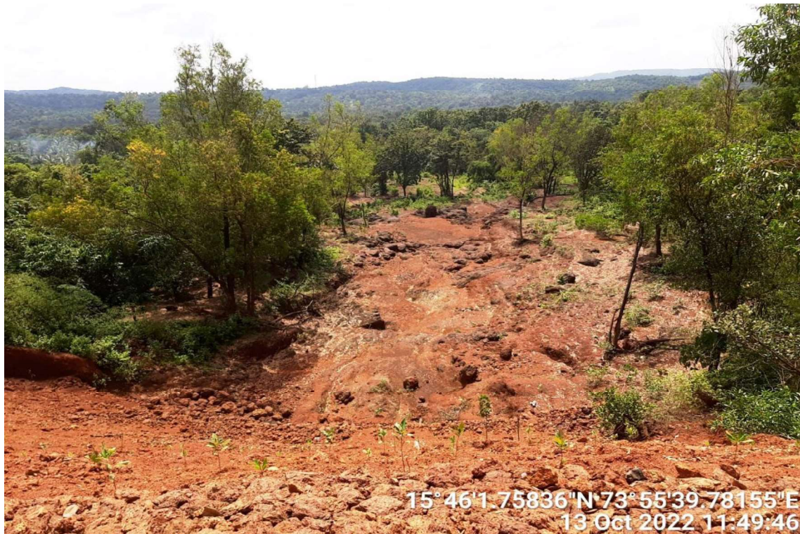
Photograph-4: Boundary of mine wall breached during the incidence, resulted in flow of mine pit water d/s to the agricultural fields.
