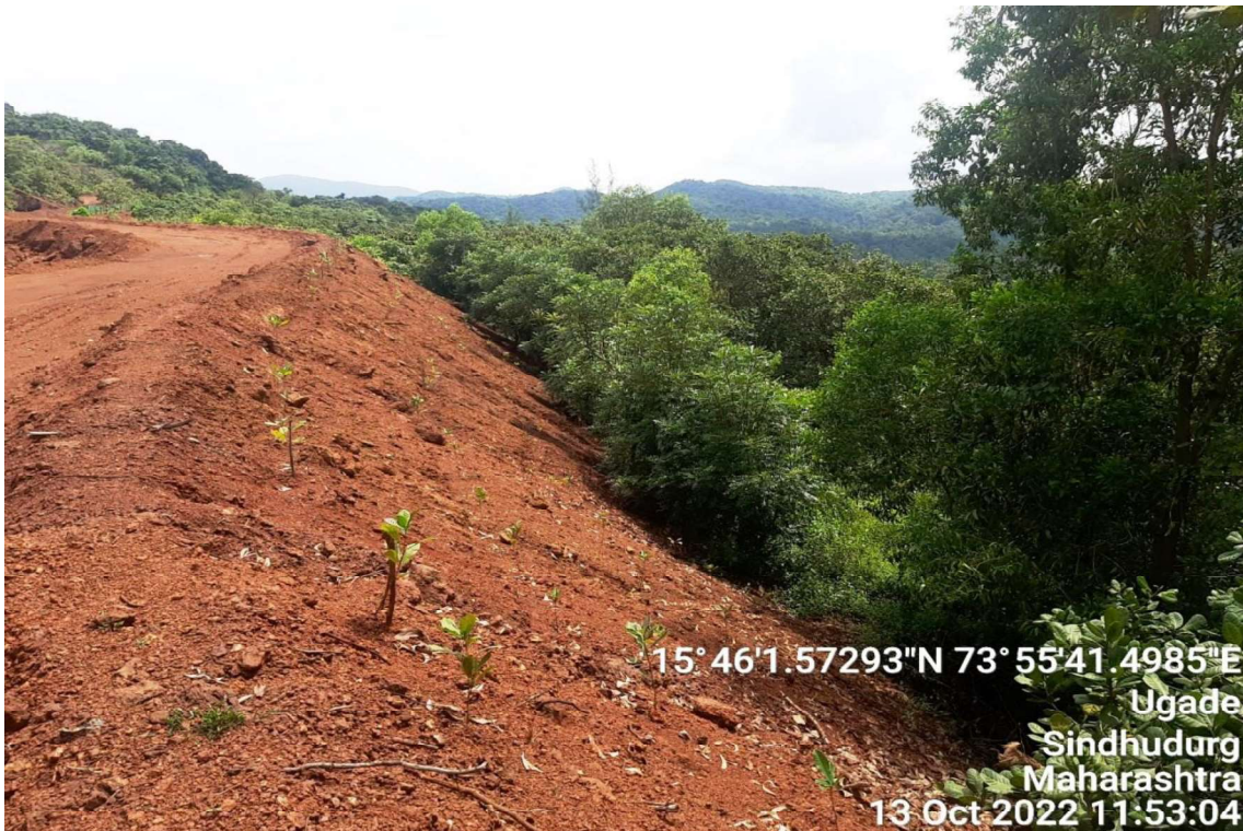
Photograph-6: Mine boundary wall augmented with overburden and plantation of cashew saplings.
