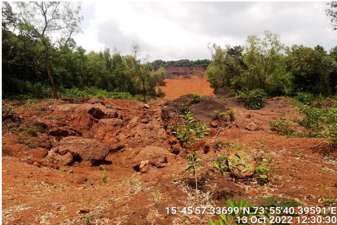
Photograph-8: A view of breach of mine wall occurred and path of flow of mine pit water towards d/s.
